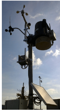
(a) The fixed weather station with the solar panel below
